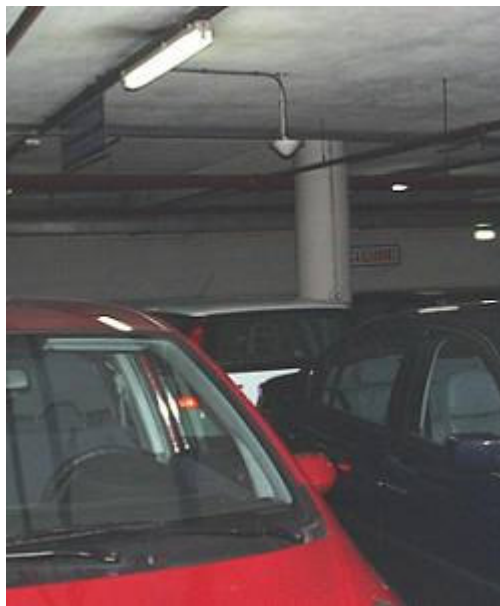
Figure 2.7 – BS antenna on a ceiling in an in-building environment.
