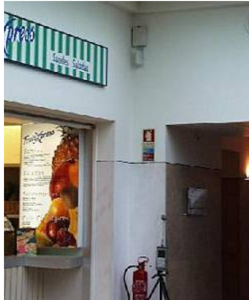
Figure 2.8 – BS antenna wall-mounted in an in-building environment.
