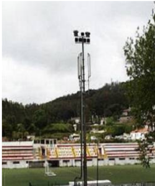
Figure 2.5 – BS antennas on a light pole in an urban environment.
